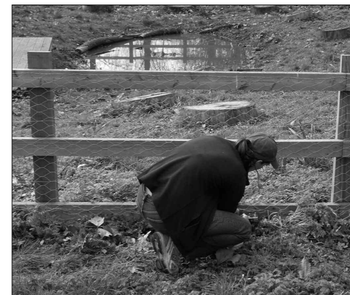
One of the friends attaching wire netting to the fencing around the pond to stop dogs from running in
