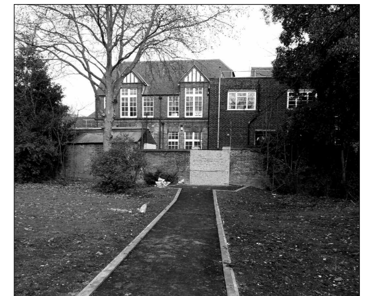
A new path, under construction from Downhills School through to Downhills Park
