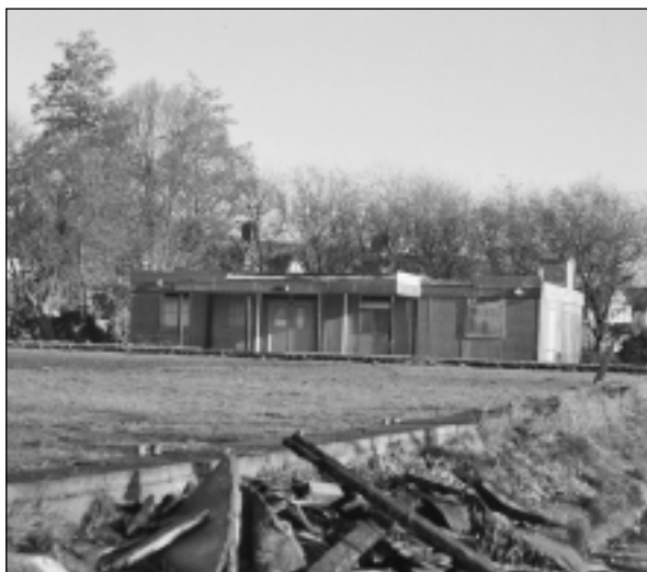
A sorry sight after years of active use. The bowling club pavillion will be demolished soon.
